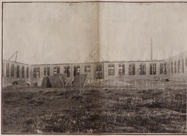
VIEW FROM OPPOSITE THE MAIN ENTRANCE NOTE THE RAPID PROGRESS OF THE WORK
